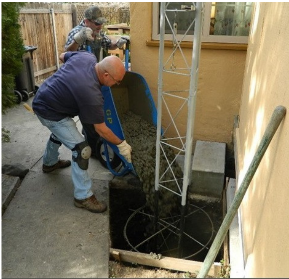
WB6JMM and KD6FVA fill the 5 foot deep hole for the antenna base.
