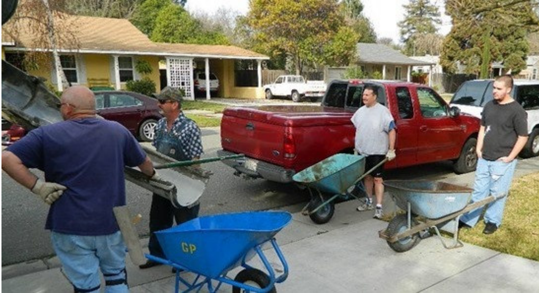
Waiting for the cement to come down the chute: Dave WB6JMM , John KD6FVA , Tom N6TMA , and helpful neighbor Jason.
