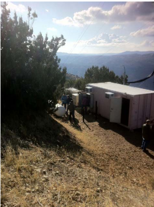
Repeater Site on Mt. Oso with vault and diesel generator.
